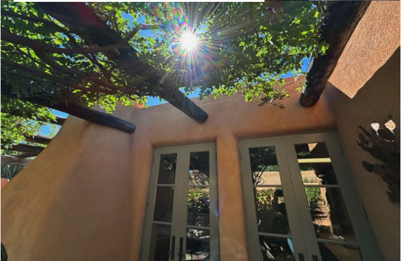
ROTTEN PERGOLA STRUCTURE TO BE REPLACED - NON-HISTORIC MATERIAL TO THE EXISTING HOUSE BUT WAS ALL RECLAIMED BARN WOOD THAT HAS STARTED TO CRACK AND BEND.
