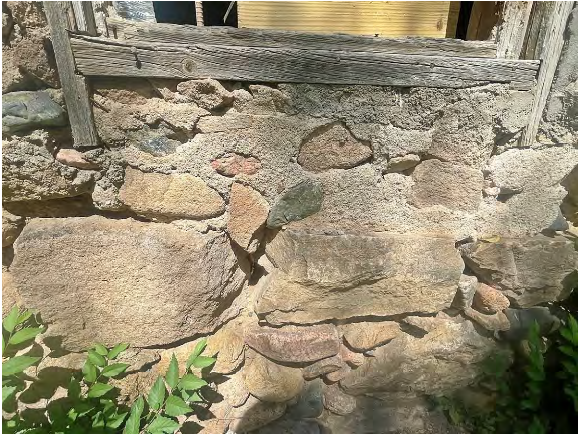
Photo 16: Stone Structure. Mortar at window opening. Camera facing north.
