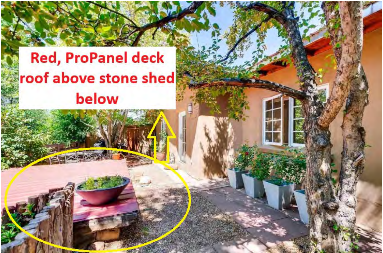
This is a picture of the south elevation from Zillow. This shows what the Backyard area looked like before Lisa Andree Falls took over ownership. The Red propanel material served as the stone shed's roof prior.
