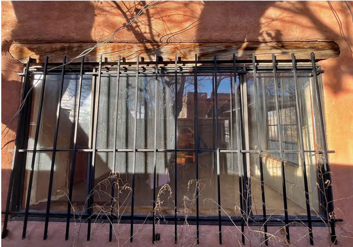
Photo 12: South elevation at 1980s addition. Window at living room. Camera facing north.
