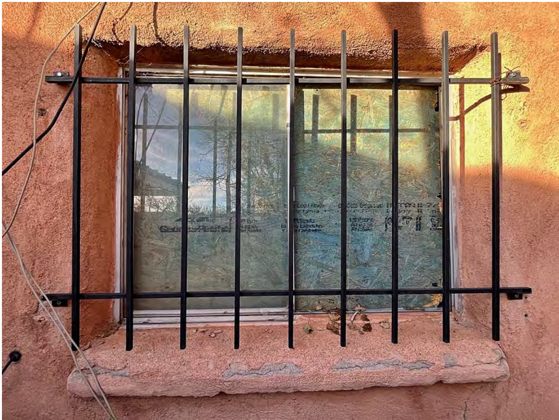
Photo 14: South elevation. Window of southeast room of the original core. Camera facing north.
