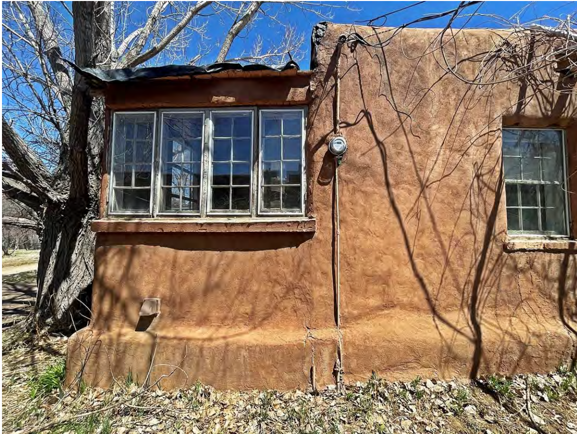
Photo 6: North end of west elevation. Post-1969 porch enclosure at left. Camera facing east.
