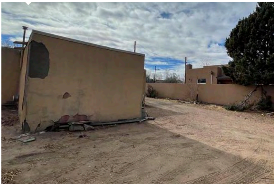
Wood framed addition – pre collapse - 2023
