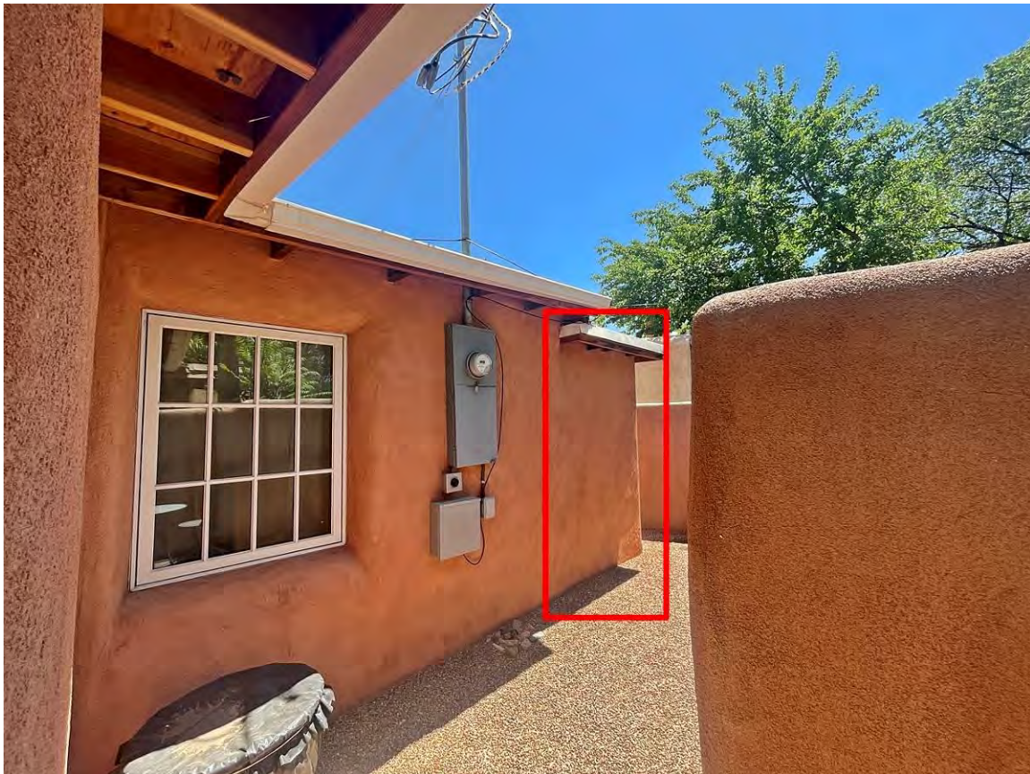
Photo 12: South elevation, east section oblique. 1970s closet addition highlighted. Note single sash casement at left.
