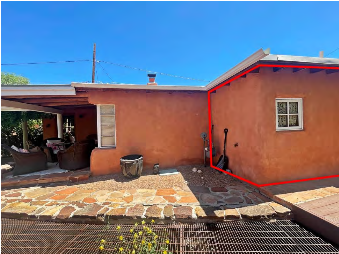
Photo 10: South elevation, west end. 1970s bump-out highlighted. Camera facing north. Note grated acequia.
